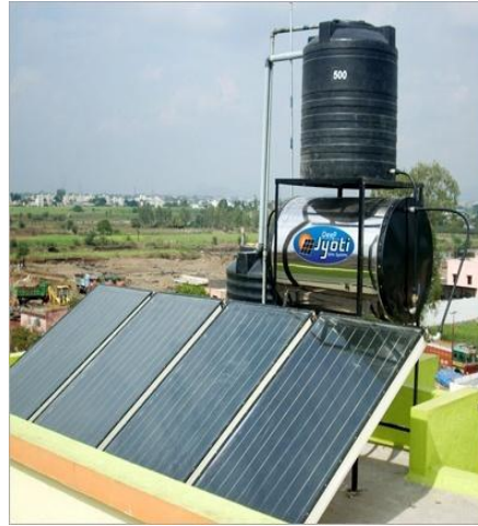
Photo 1. Flat Plate collector
